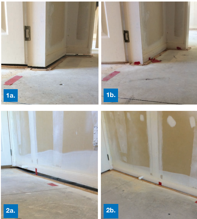
1a, 2a: Before and 1b, 2b: After Teretek® engineered resin being injected
