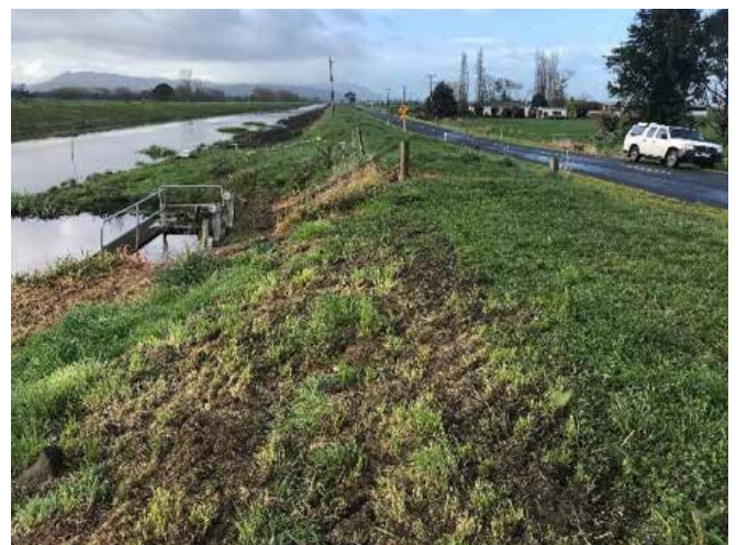
The culverts ran beneath a road frequented by heavy milk tankers, further exerting pressure on the sinking structures.
