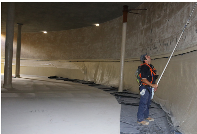
Mainmark technician applying polyurea product on the wall of the water tank
