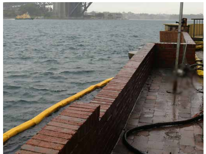
Filling the voids behind the sandstone blocks, re-supporting the seawall, and lifting and re-levelling the patio area
