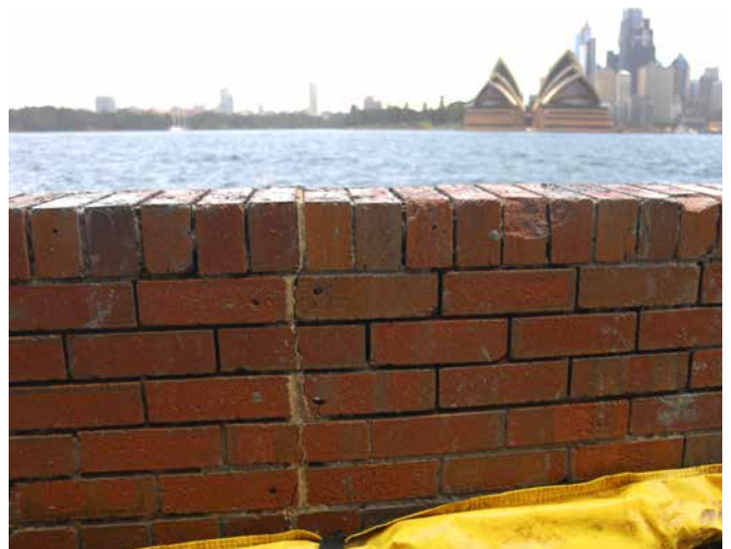
Cracks in sea wall of the property due to continuous water movement, subsidence and erosion
