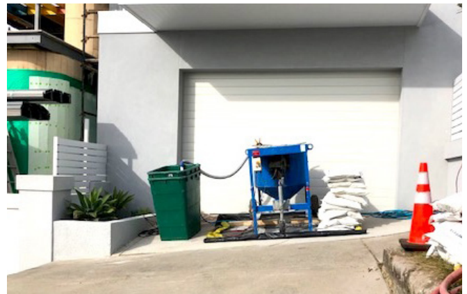
Mainmark equipment set up outside the home, with minimal disturbance and occupied space
