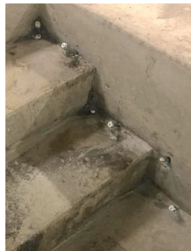
Water leakage through basement staircase after injection
