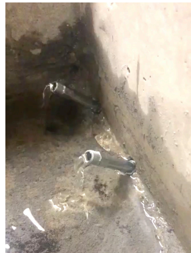
Water leakage through basement staircase before injection
