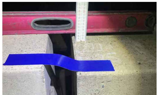
The Mall bridges' subsidence was most clearly seen in the variation of levels on the pedestrian walkway walls.
