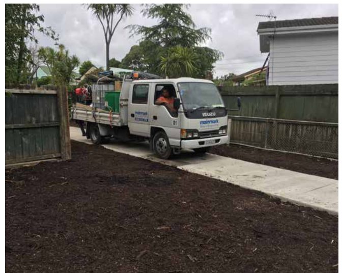
Access to pumping locations was limited so Mainmark planned carefully to avoid significant disruption to the public parkland.
