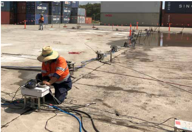
SEQH needed to find a solution to remove dishing and water pooling along the hardstand's midline (seen in the background)
