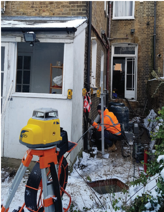
Mainmark Technician injecting Teretek® engineered resin, using a laser level and receivers to monitor the accuracy of the house lift
