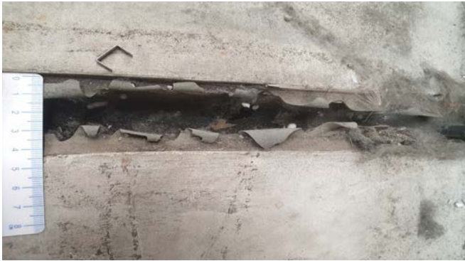
Large crack in floor between concrete slabs
