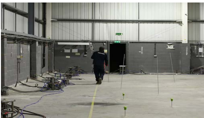
Rear corner of site experienced significant subsidence
