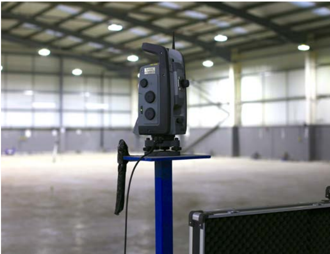
Trimble stations monitor and record level data during re-levelling
