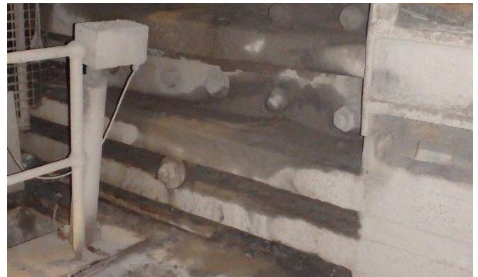
The oil bath surrounding the crusher needed to be removed before Mainmark solution could be applied
